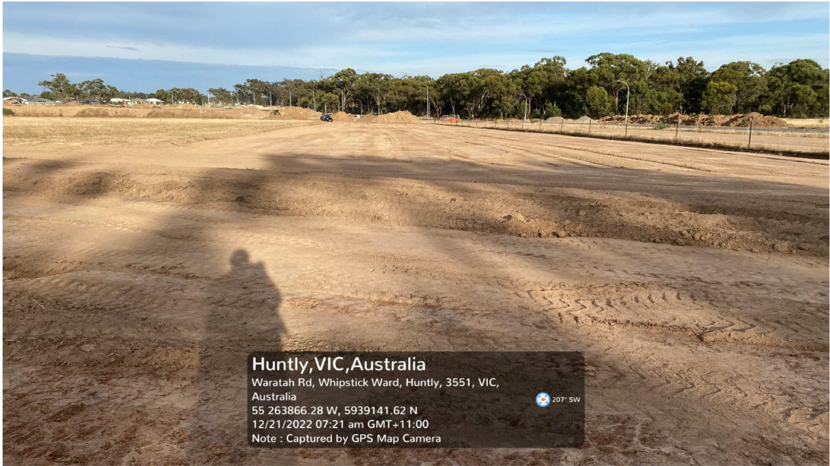
P1: General view of Stage G1 (the pipe and covering soil was removed and inspected at a later date)
